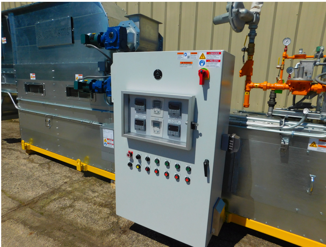
Control Panel Assembly
